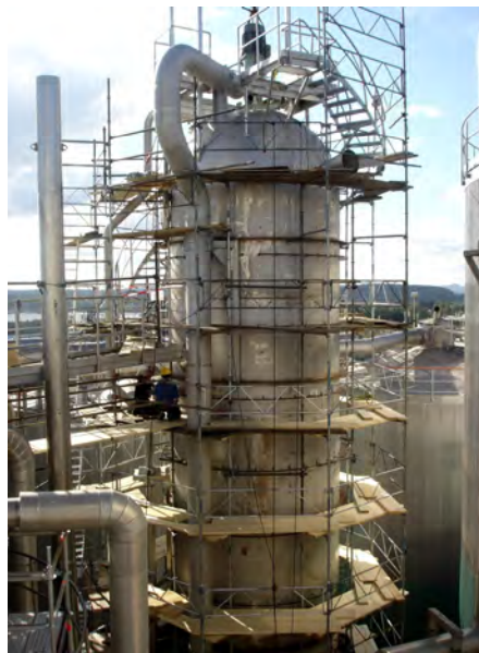
Figure 12.6. Hydrogen peroxide reactor in LDX 2101 ® , constructed in 2006
