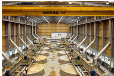
Figure 12.11. Embedded leach tanks in a zinc plant, installed in duplex 2507
